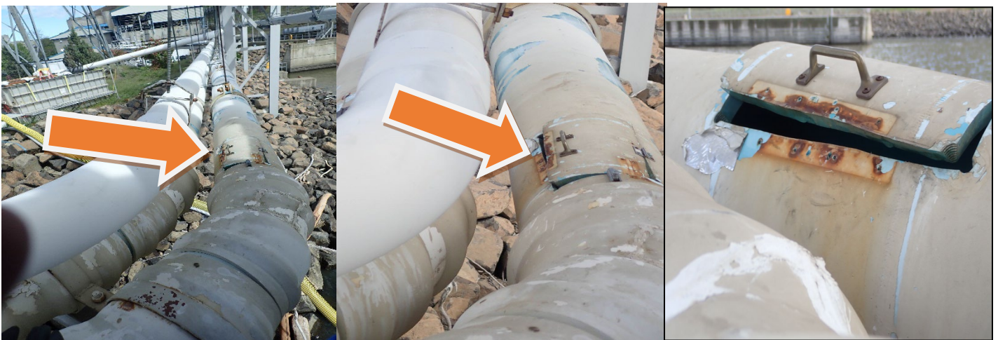
Cleanout hatch condition leading to incident
